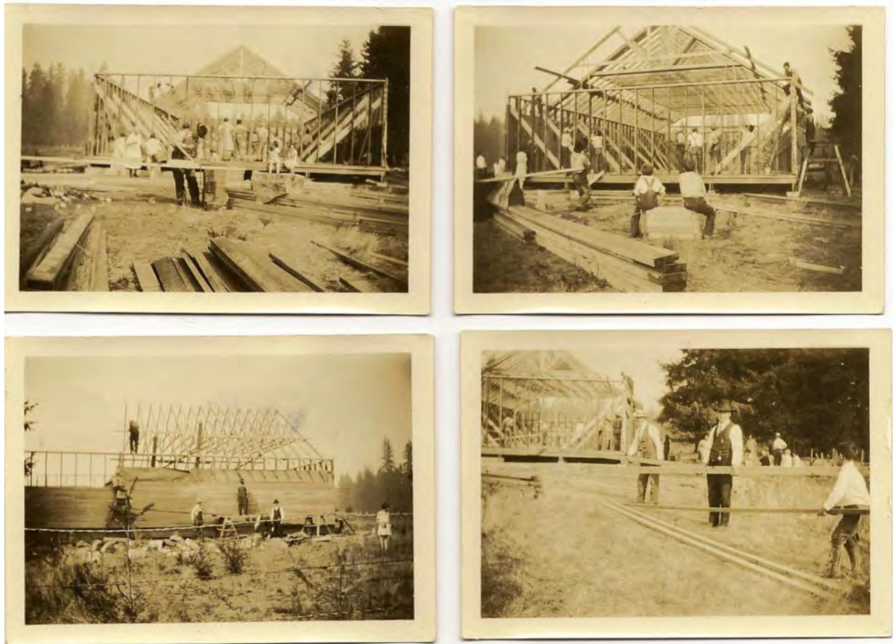
Figure 5.67: Elk Plain #782 in Pierce County, ca. 1927 (Members and community volunteers constructing the hall, courtesy of David Bryant)
