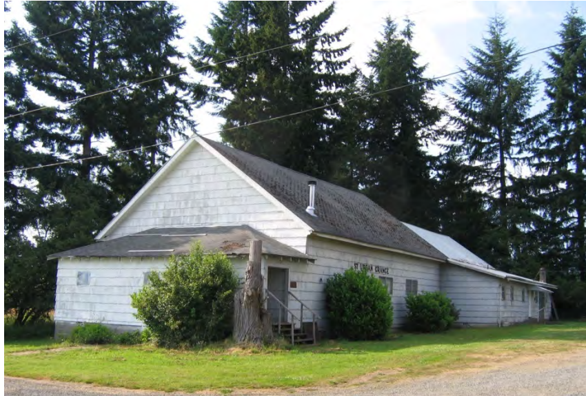
Figure 7.9: St. Urban #648 in Lewis County (Example of former community club adapted for use as a grange hall, with kitchen rear addition)
